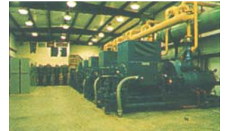
Inside, water and air are cooled and pressurized
